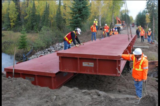
Photo 2: 90 Ton capacity crane lowers section 2 (downstream of Como Lake) into position. MTO Construction crew workers guide section to line-up with section 1.
