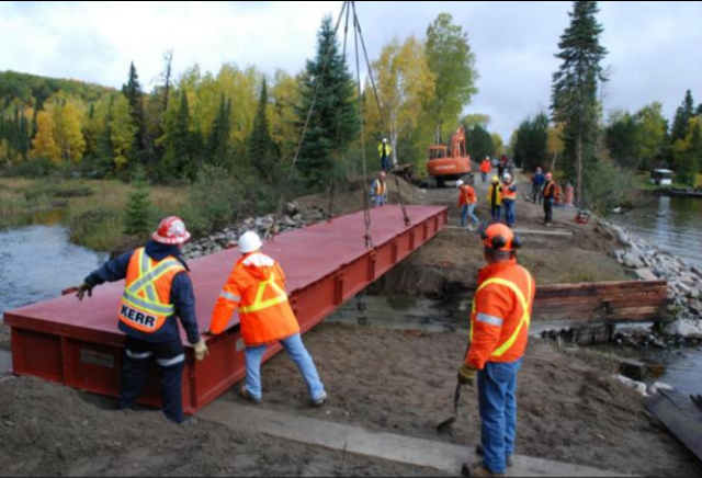
Photo 1: 90 Ton capacity crane lowers section 1 (downstream of Como Lake) into position. Old bridge has been removed, new concrete bearing surface is visible at both ends.
