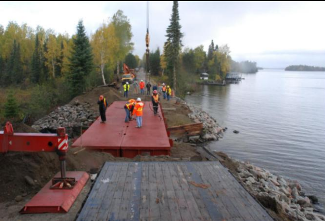
Photo 3: Section 1 and 2 of 18.3m span Lessard Modular bridge are both in final position. Crews disconnecting overhead crane lift cables.
