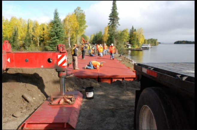
Photo 4: With section 1 and 2 in position, MTO construction crew attach bridge section together at tie-down points using structural bolts with washers and nuts.
