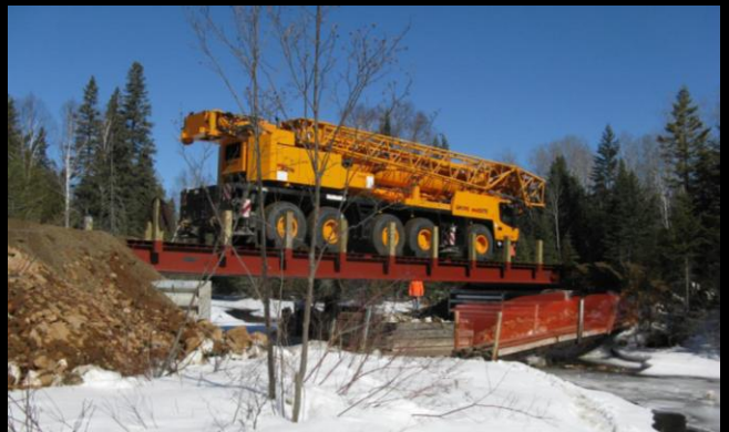
Photo 6: 90 ton capacity crane crossing new Como Lake bridge enroute to Bass Lake (another MTO - Lessard Welding bridge project).
